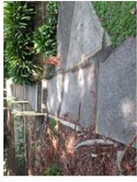
D. Existing Paths Maintain (mostly) existing paths and repair any trip hazards.
