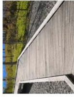
F. Boardwalk Elevated boardwalk to provide safe connection over water runoff area.
